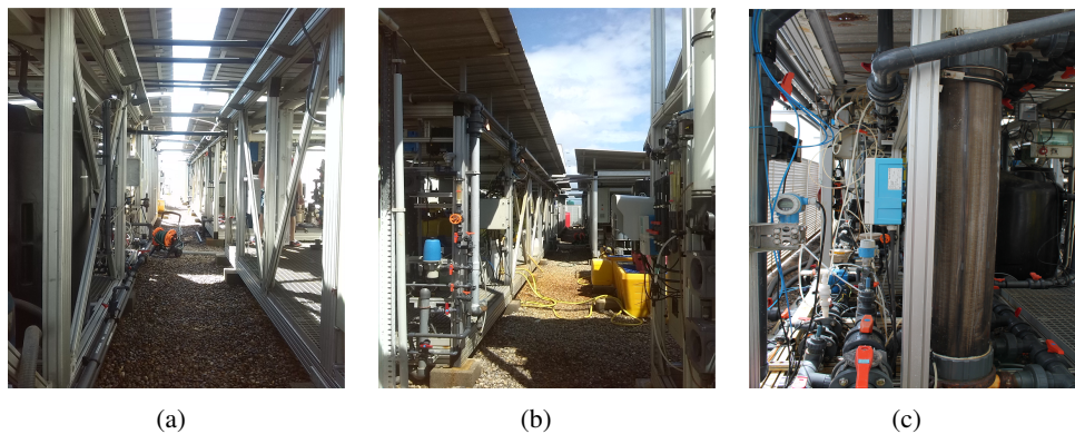
Fig. 15. La Tordera's water desalination pilot plant.
